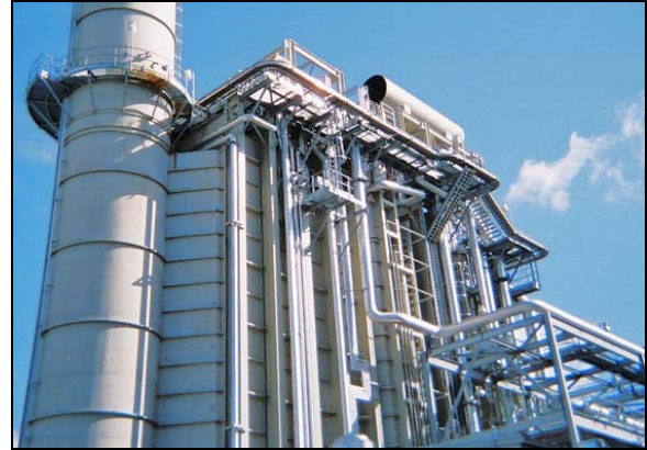
Figure 6: Heat recovery steam generator showing surface clutter in the form of structure, piping, and platforms that scatter and diffusely reflect much of the incident acoustic energy.
