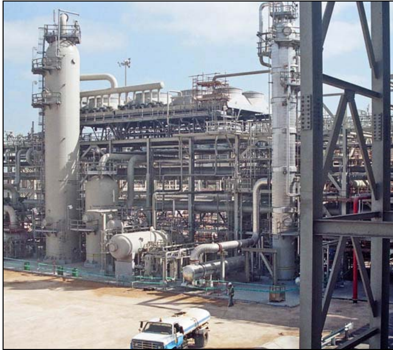
Figure 8: Very large pipe rack with air coolers on the top that scatters, diffusely reflects, transmits, and diffracts incident sound.
